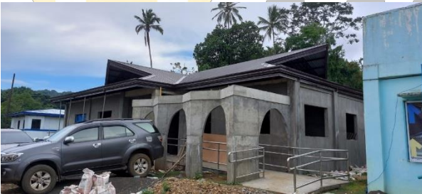
This is the under-construction site of Bayang Rural Health Unit. Photo source. Mine
