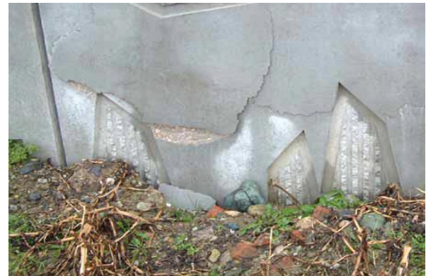
Fig.3. Deterioration due to freezing
